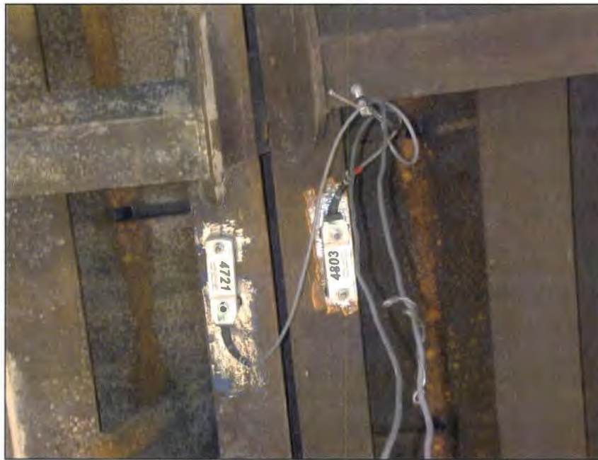
a. Strain transducers 16 and 17 on bottom flanges of girders at LFC
